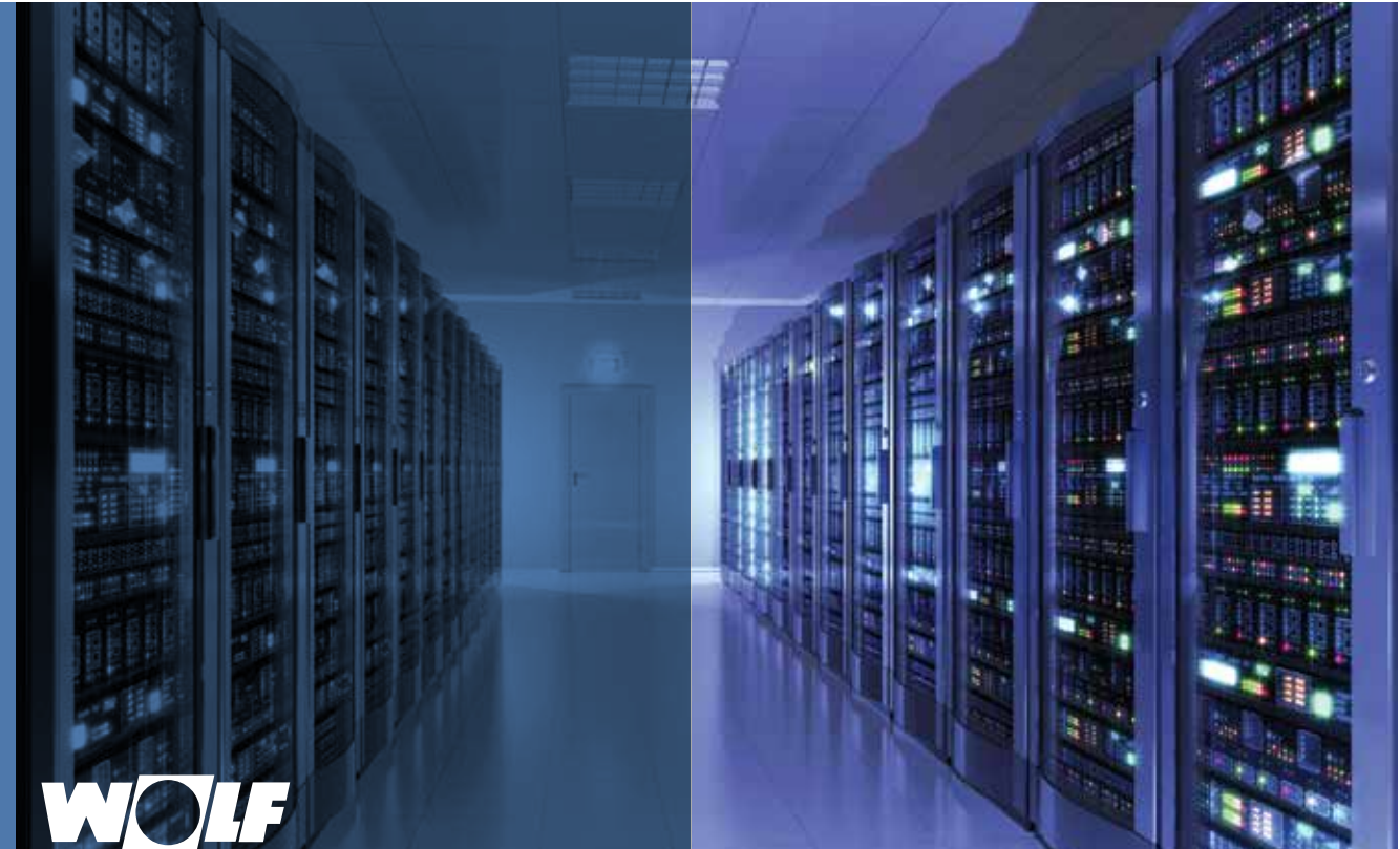
Precision Air Conditioning System
